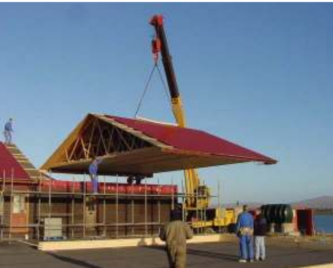
space. The roof being lifted from the SEAFISH Chandlery for the new construction of an upstairs office. It was replaced the day. All photos by Penguin News except where shown.
