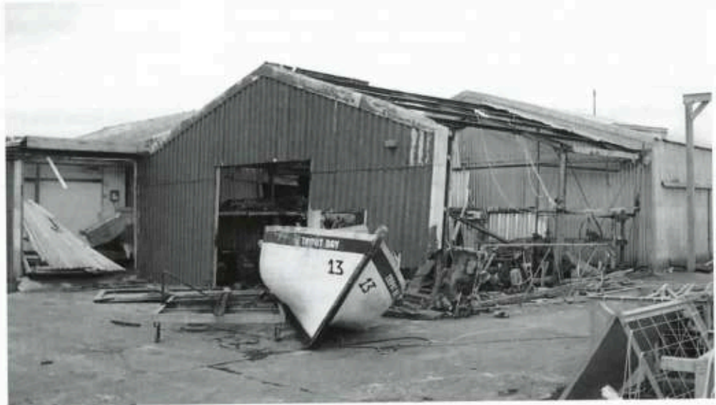
Above: The fish factory on Tristan damaged in the storm
