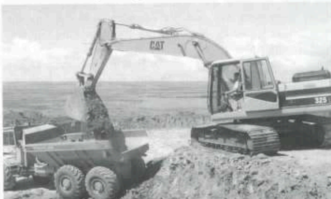
Road building material being loaded by the East Falkland road gang as it pushes the North Camp road onwards towards Cape Dolphin.
