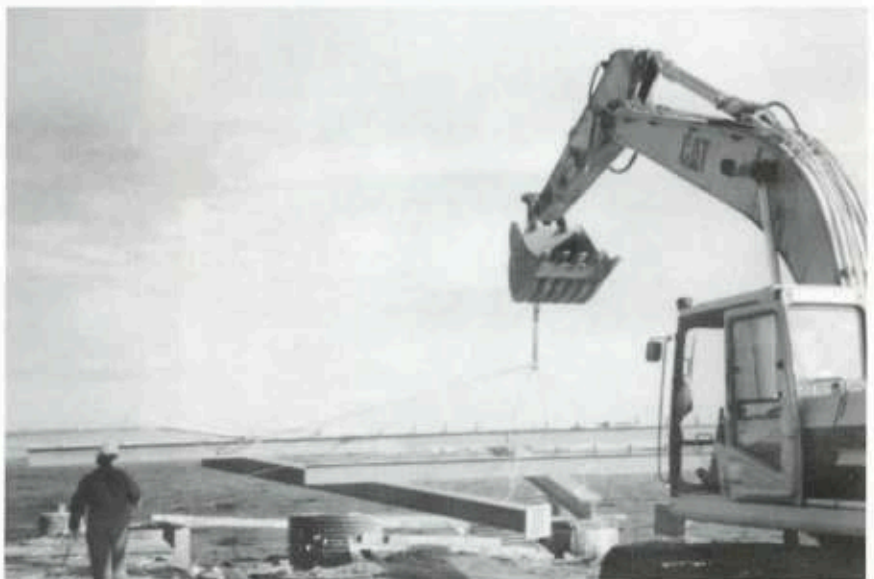
Steel work being lifted into position. This is used to link the causeway and the berth and will in due course be timber decked. Photos: M. Young
